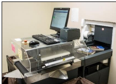
Behind the scenes view of the book sorter equipment behind the book drop
